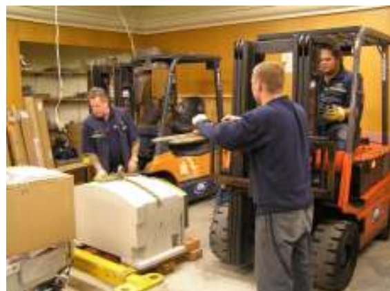
Grouting in the baseframe and the new Varian iX linac gets delivered
